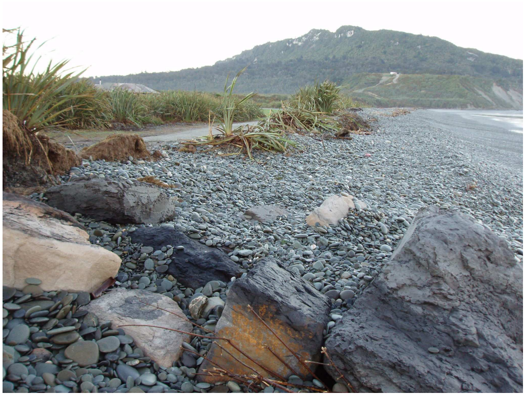
Figure 6: Breached gravel barrier and overwashing of gravel on to the Esplanade immediately south of the end of the rock revetment at Stathan Street (August 2006).
